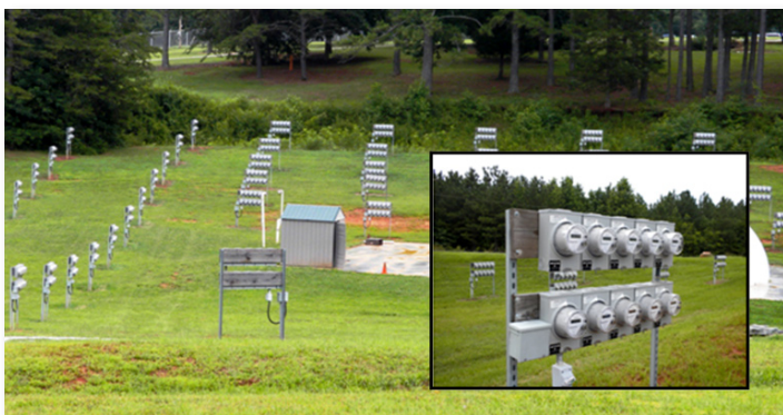
Figure 1 – Meter farm at the manufacturer’s facility with a rack of 10 smart meters in the inset.
